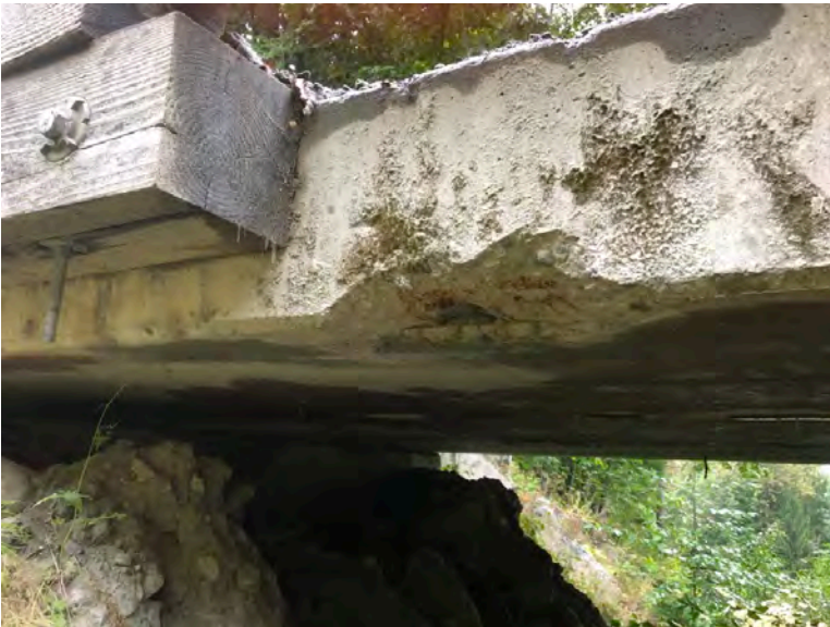
Minor slab damage upstream
